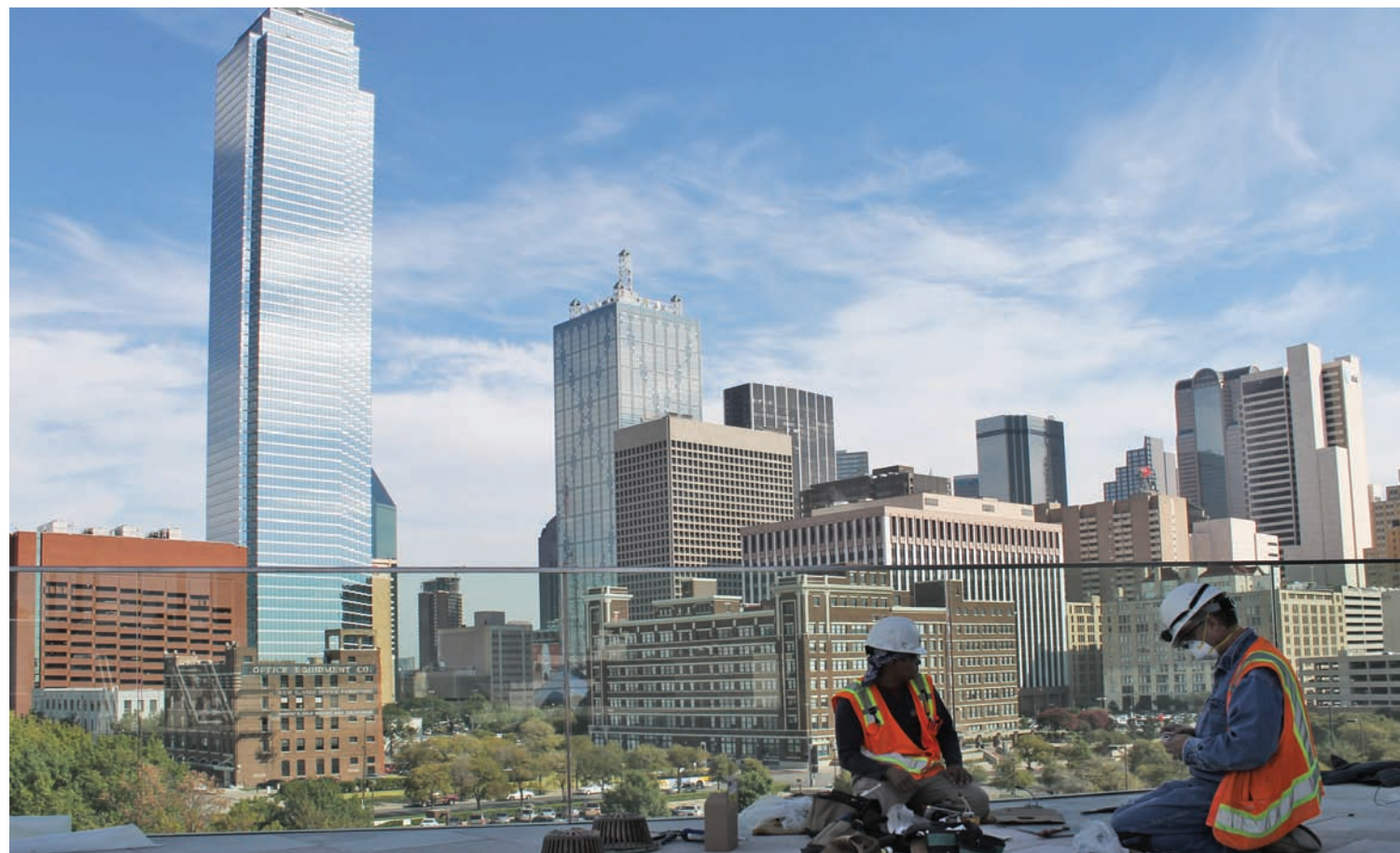
ROOMS WITH VIEWS | Workers put the finishing touches on the outdoor pool deck this week at Dallas' convention center hotel, as the downtown skyline looms behind them. The hotel is scheduled to open Nov. 11. (John Wright/Dallas Voice)
