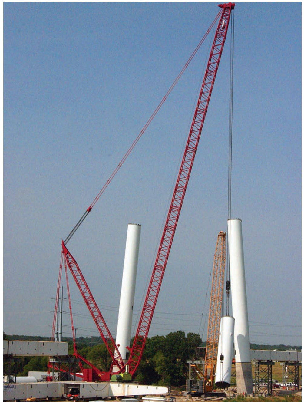
BRIDGE WORK | Workers use a crane to lift a piece of the arch into place on Thursday, June 3 as they continue work on the Margaret Hunt Hill Bridge. (David Taffet/Dallas Voice)
